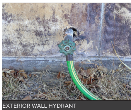
NO FIRE SUPPRESSION IN KITCHEN HOOD
