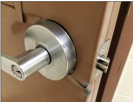
DAMAGED DOOR AND PANELS
